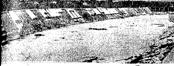
REPAIR WORK---Patches of new concrete stand out in contrast to the old wall of the almost-empty flume north of the siphon bridge.
