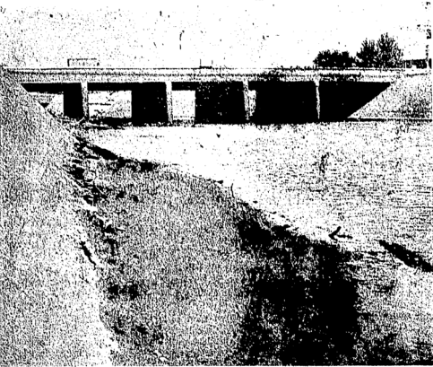
LOW WATER---The stream bridge looked like just any other bridge across a stream as they emptied the flume to effect major repairs on the structure during the past week. Take a good look---the flume isn't empty very often, and this repair job should last for a long time.
