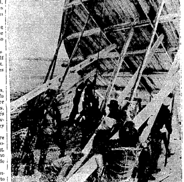
Construction of rural buildings with native materials has gained great interest in Michigan. This shows a barn raising near Fairview, Michigan State college is offering a new short course in rural building.
