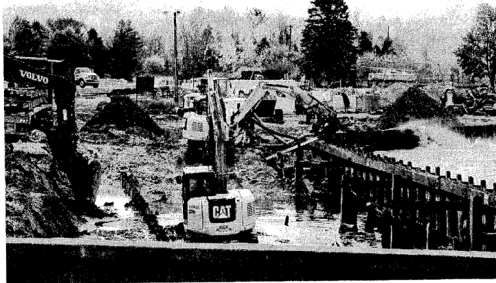
Pioneer Tribune file photo Contractors struggled against the high water levels of Lake Michigan this summer while working on the Manistique Marina update.
