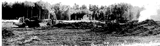
Above, logging has been taking place along Highway M-149, approximately one mile north of U.S. Highway 2, to clear the land needed for a new hatchery building and six rearing ponds for the production of walleye and muskellunge as part of an update and expansion of the Thompson Fish Hatchery.
