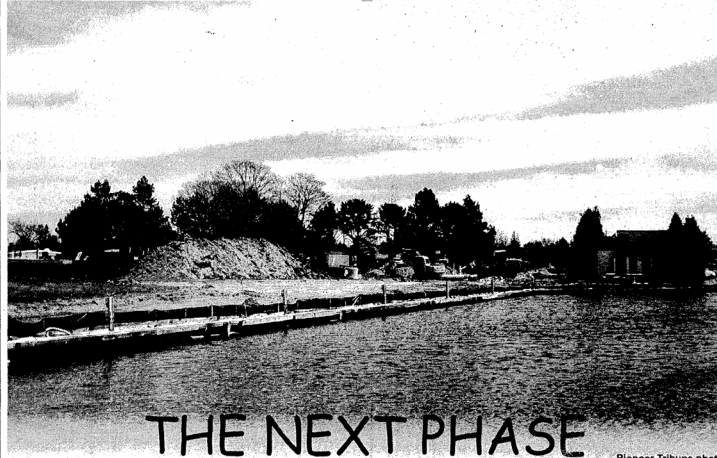
Construction on the Manistique Downtown Development Authority's third phase of marina updates has begun. The project includes an updated parking lot on the eastern half of the marina, new sidewalks, new electric and water service, lighting upgrades, and the installation of new, floating docks. The portion of the marina roadway that goes beyond the parking lot will be removed and made into green space and new walkways and railings will be installed around the docks. Work will continue through the summer until the end of October.
