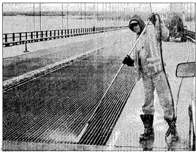
Courtesy photo of Mackinac Bridge Authority employees sweeping and washing off sand and road salt that is tracked onto the bridge and accumulates in nooks and crannies each winter.
