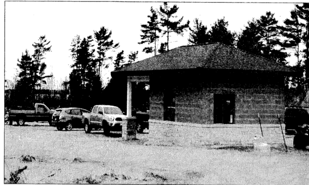
Pioneer Tribune photo The Manistique Lakeshore Campground continues to take shape, with construction crews on site Wednesday morning to work on the property. The campground is slated to open sometime in June.
