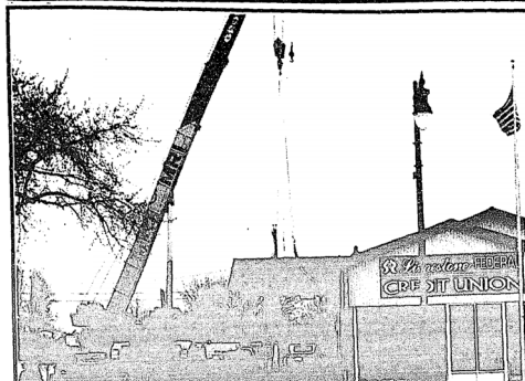
Limestone Federal Credit Union broke ground last week on their new building — a facility expected to provide greater security, more convenience and privacy for customers, more stations for conducting business, more parking and other amenities. The project is expected to be complete this fall. Above: Workers remove the canopy over the old drive-through lane. (Pioneer-Tribune photo)
