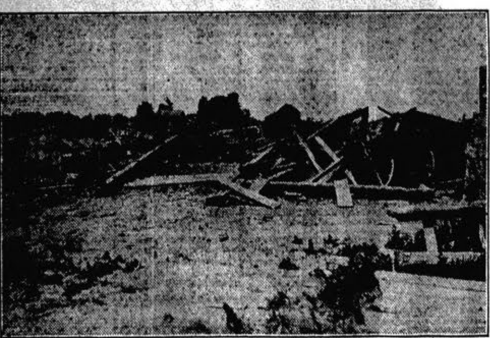
AFTER THE STORM—This shows what is left of a fine hewn-timber barn, 30x40 feet, belonging to Sherman Fluor, Section 31, Grant Township, Cheboygan County, destroyed by windstorm June 22, this year. It is a TOTAL LOSS—NO WINDSTORM INSURANCE! Can you afford to have this happen to you?
