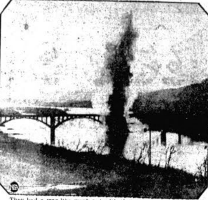
They had a war-like work-out with their aerial bombs did Army airmen when they razed this concrete bridge erected for experimental engineering across the Pee Dee river in southern North Carolina. The moment of detonation of one of their big winged pellets of destruction is caught by the camera here.
