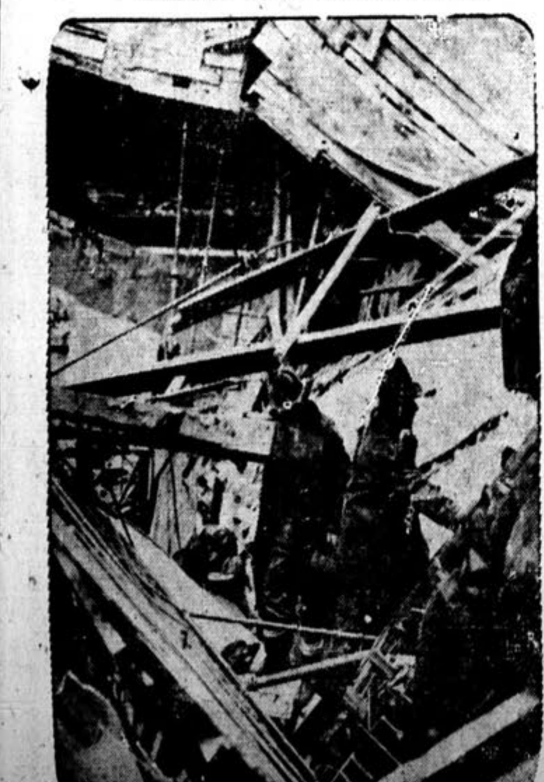
Several workmen were injured when the Parker House, Boston, birthplace of the Parker roll, collapsed during its demolition. Photo shows firemen searching for injured.
