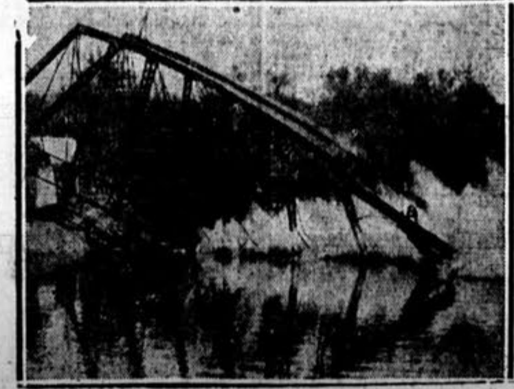
AND DOWN WENT THE BRIDGE! —This is not the famous London bridge falling down, but one near Cincinnati. And its collapse was intentional. Acetylene torches cut through the supporting steel beams and 170,000 tons of steel fell down into the river. The bridge was destroyed to make way for a new one. It spans the Little Miami River at Milford, O.
