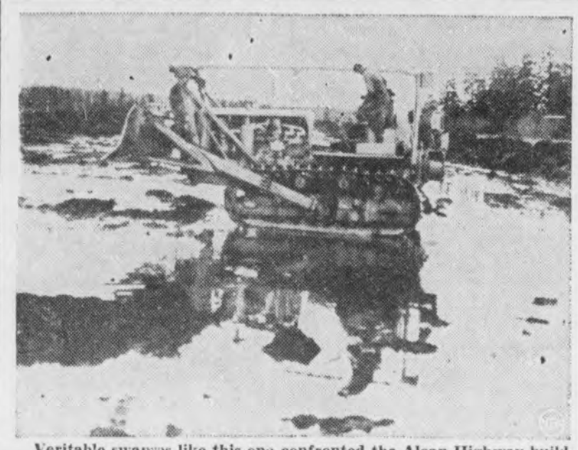
Veritable swamps like this one confronted the Alcan Highway builders pushing through treacherous muskig areas along sections of the projected road.
