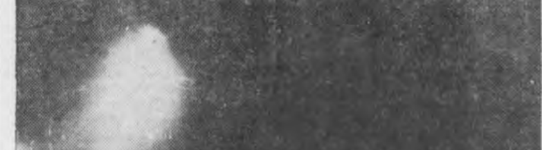
With need for power for war industries, work on Shasta dam near Redding, Calif., is being carried on day and night. About 200,000 cubic yards of concrete are being added to the structure each month. This night scene shows construction being carried on.
