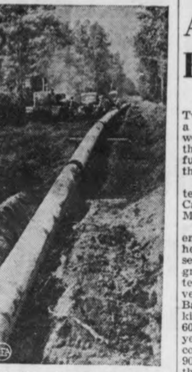
Wartime demands for oil in eastern U. S. rushed construction of Plantation Pipeline to carry gasoline from Louisiana to North Carolina. Piece of pipeline is shown being lowered into three-foot trench that hides it from air attack.
