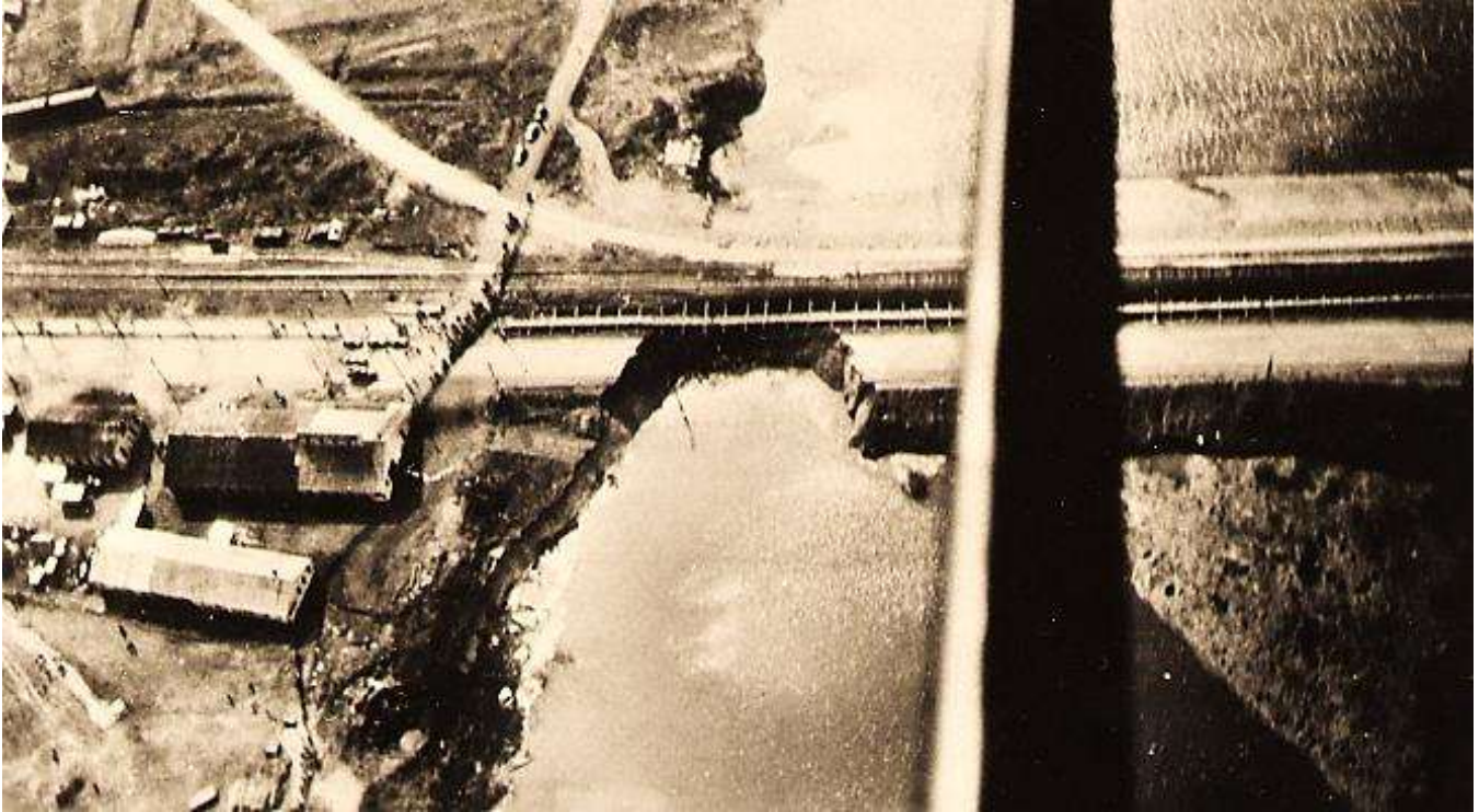
This aerial view, taken sometime after May 3, 1940, shows the missing portion of the highway crossing the Chapin Pit in Iron Mountain. The Chapin Mine shops are visible at the lower right. [William J. Cummings]
