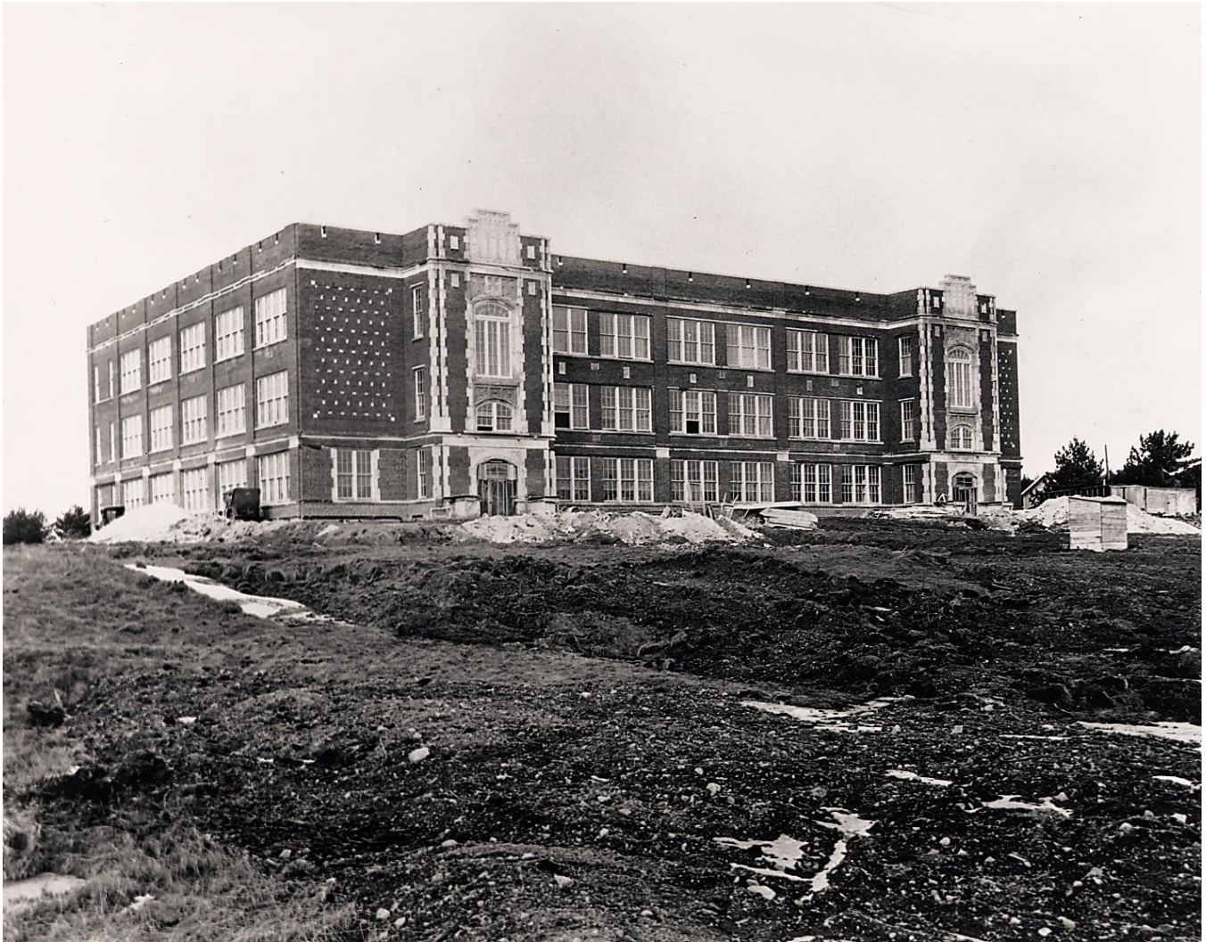
Edward G. Kingsford Junior High School (Kingsford High School), Hamilton Avenue, Ford Addition, Kingsford, 1925: Kingsford Junior High School was rapidly nearing completion in mid-April, 1925, when this photograph was taken. Despite its name, the building served as Kingsford High School from 1925 through the spring of 1965. [Menominee Range Historical Museum]
