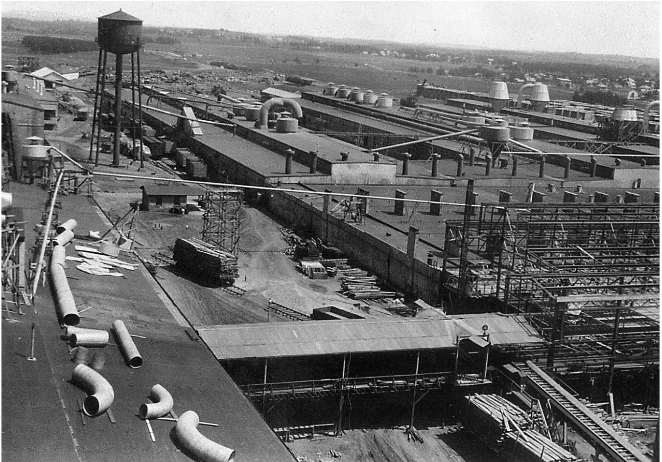
Ford Motor Company Body Plant Under Construction, Kingsford, August, 1924: This early view shows the body plant under construction. Note the horizontal flue pipe on the roof at the left awaiting installation. Waste heat was siphoned off of the power house and used in the kilns for drying, and in the Distillation and Carbonization Building for wood processing. [Guy Forstrom]
