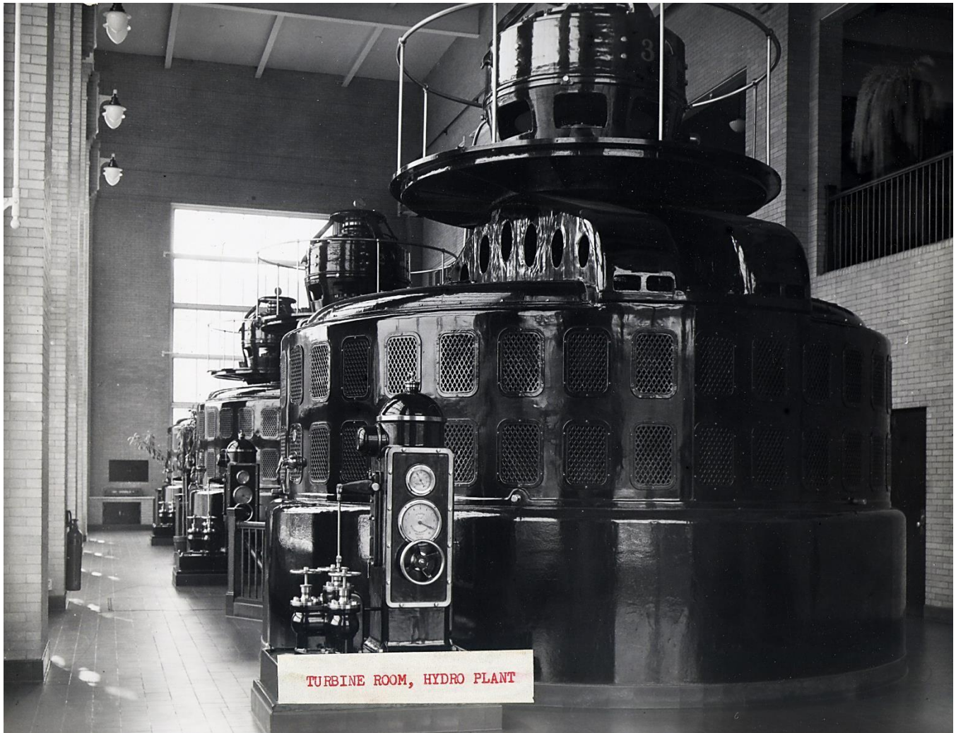
Ford Hydro-Electric Plant on the Menominee River, Turbine Room, Kingsford, ca. xxxx: [Menominee Range Historical Museum]
