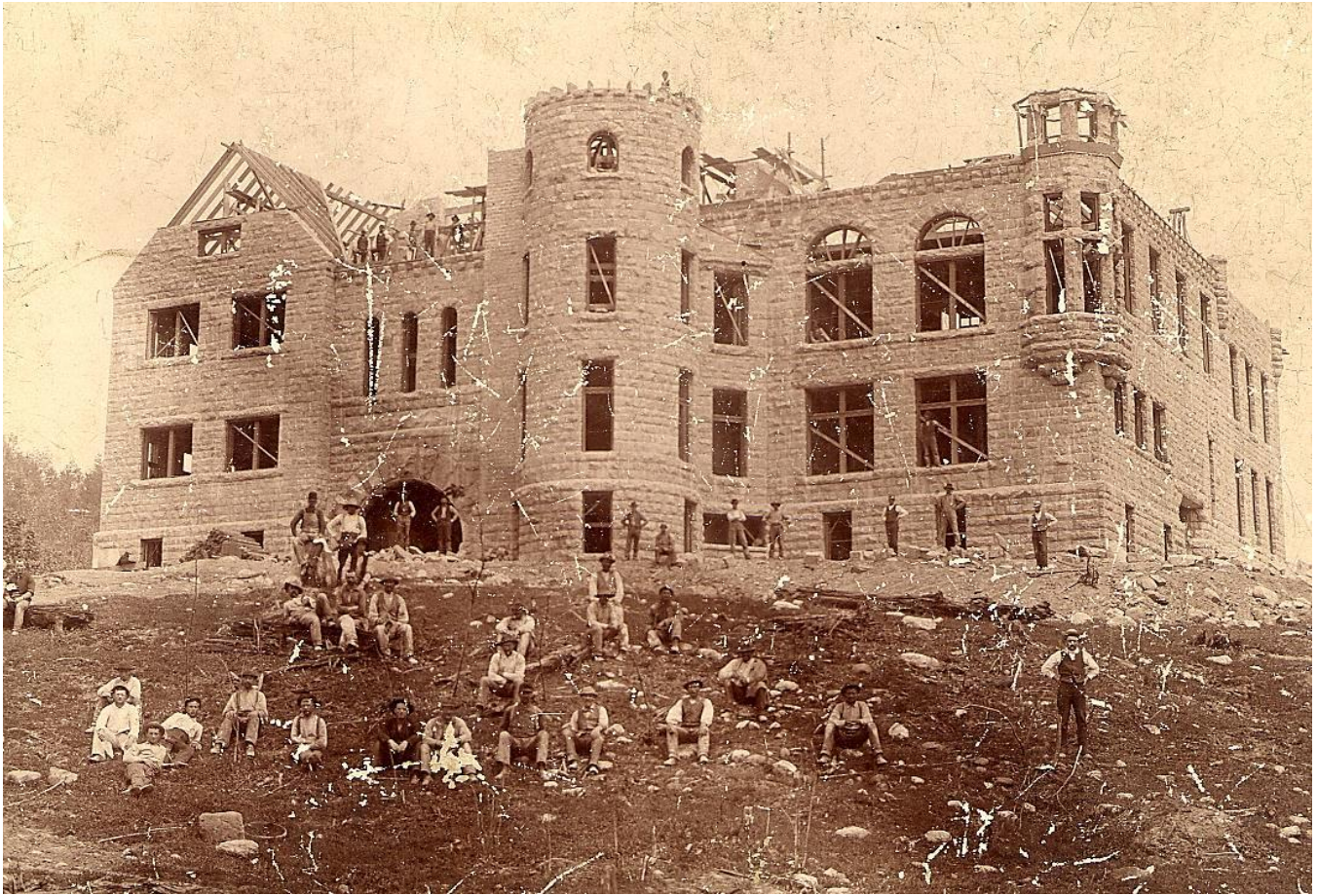
Nelson P. Hulst High School Under Construction, Madison Avenue, Iron Mountain, 1892: The Nelson P. Hulst High School was under construction on Madison Avenue at the top of East Ludington Street when this photograph was taken by Iron Mountain photographer Jorgen J. Eskil in 1892. The walls were constructed of gray granite from Amberg, Wisconsin, each block fitted and numbered at the quarry. Notice the workmen posing for the photographer. [Menominee Range Historical Foundation]
