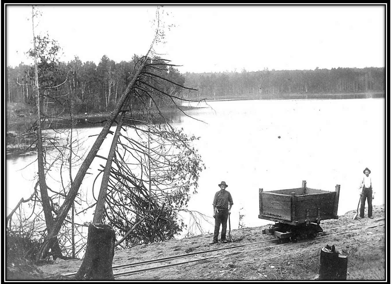
Railroad Construction, South Lake, Spread Eagle, Florence County, Wisconsin, ca. 1880: This photograph was probably taken by Jorgen Johansen Eskil, pioneer Menominee Iron Range photographer, on the shore of South Lake in Spread Eagle in about 1880 when the railroad was being built. [Menominee Range Historical Museum]
