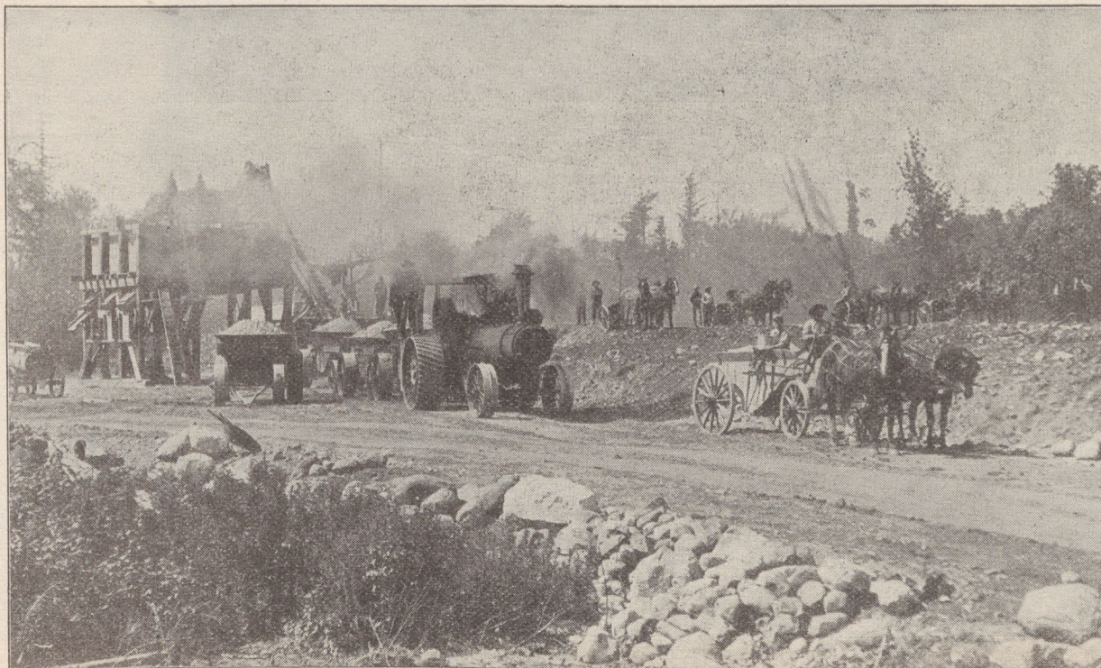
The Modern Method of Constructing Good Roads in Cloverland. Equal to the Roman Methods and Much Quicker
