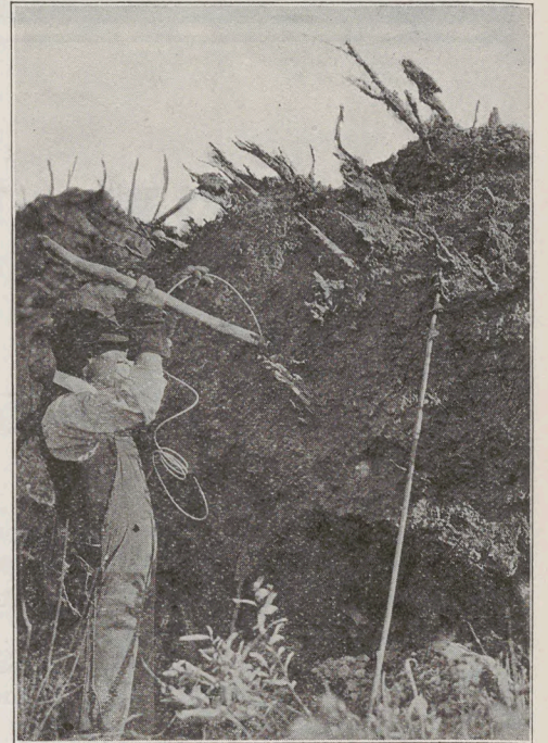
Stumps too heavy to be piled after being pulled are split with dynamite
